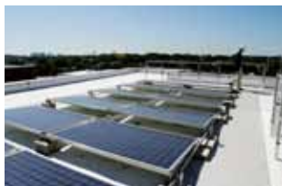
Solar rooftop at SGH
